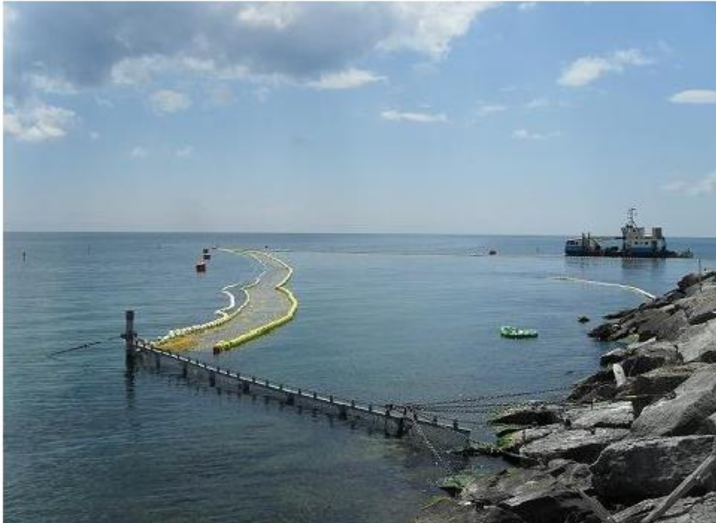
Figure 2.4: Photo of Installed Fish Diversion System from the East Side Looking West (OPG, 2012h)
